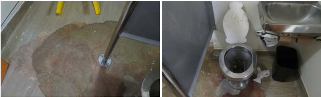
Figure 1. Damp flooring and a broken toilet in the high security facility
