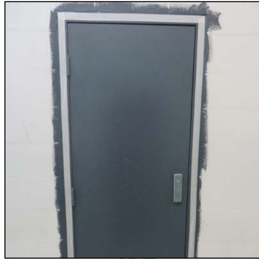
Figure 2. Repainted door in a high medium security unit
