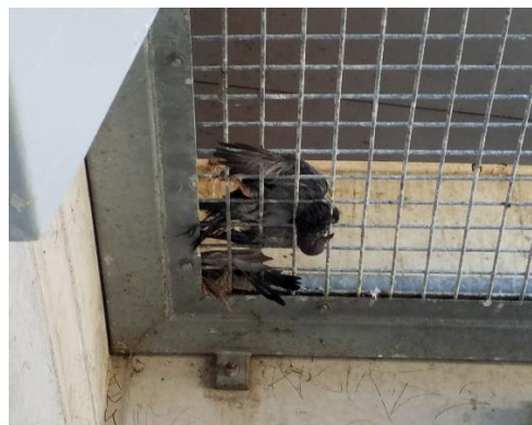
Photo 4: Pigeon carcasses caught in overhead mesh wire.
